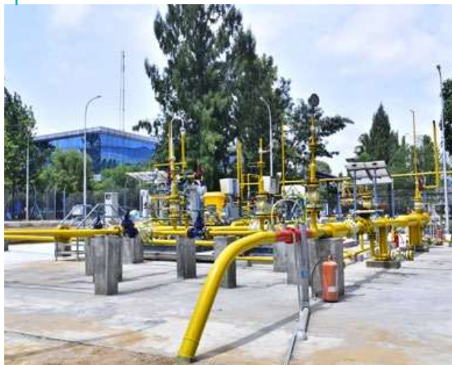
The Gail-LNG line at the Industrial Ceramics factory, Hosur
